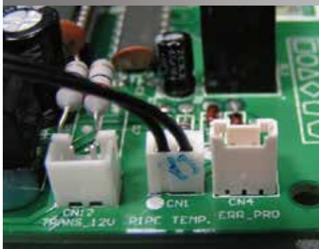
Compressor current protection
